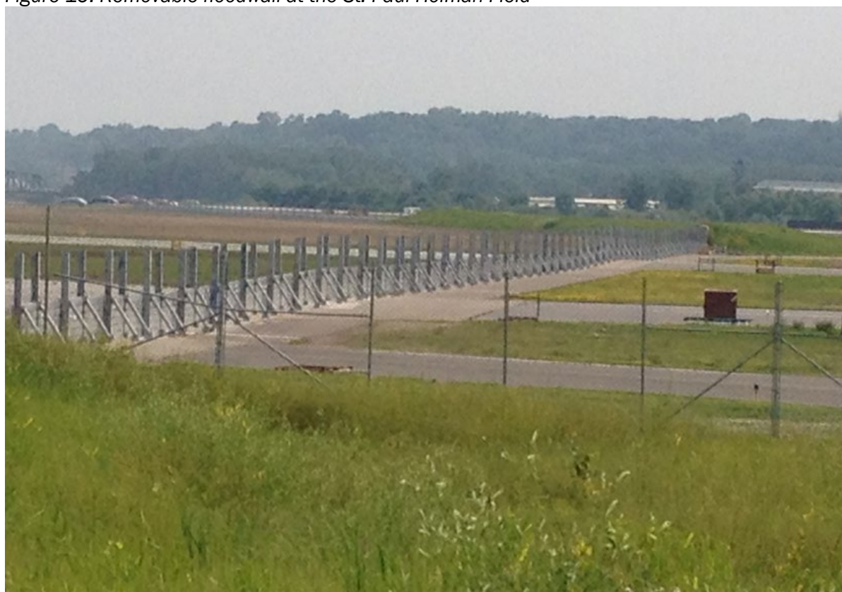
Figure 19. Removable floodwall at the St. Paul Holman Field
